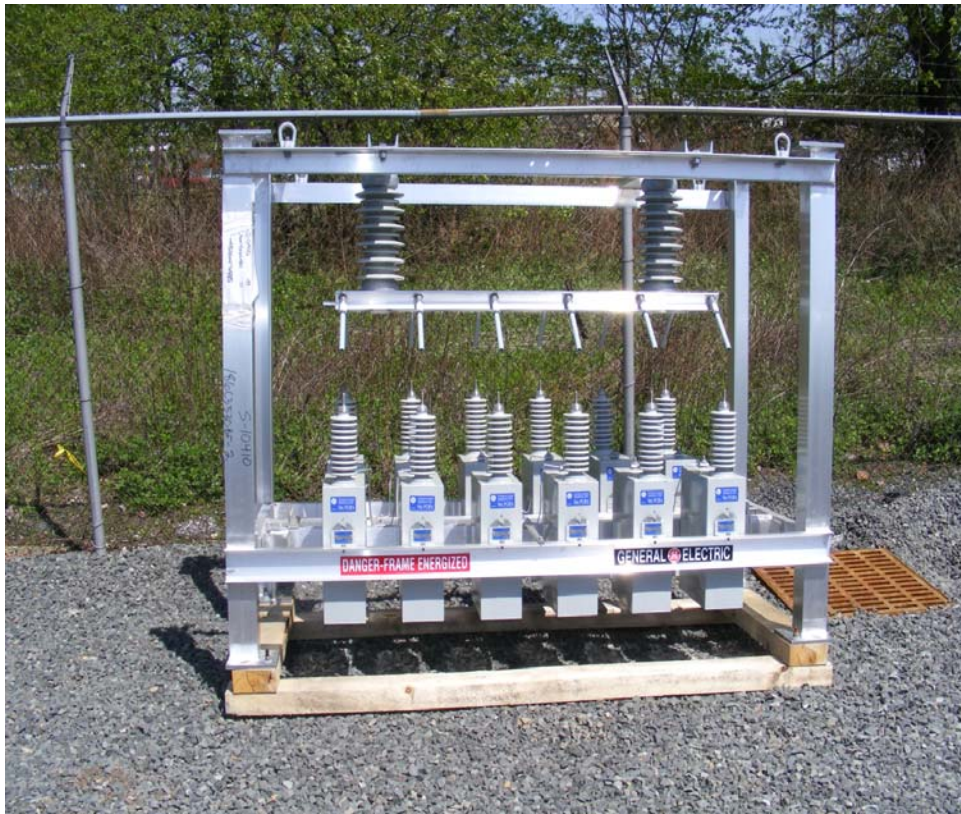
Fig. 4 - One Phase of 26 kV Capacitor Bank
