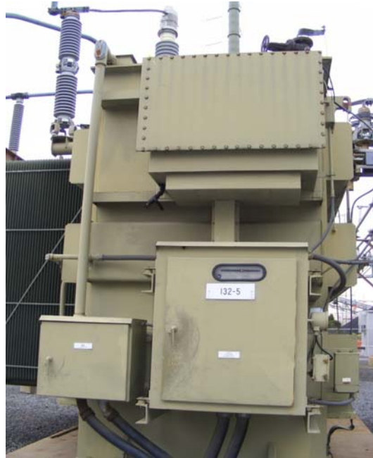
Fig. 13 - 26 kV LTC on 230/26 kV 55 MVA Transformer
